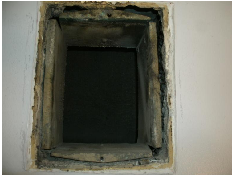
Large Gaps Around Vent Boot
