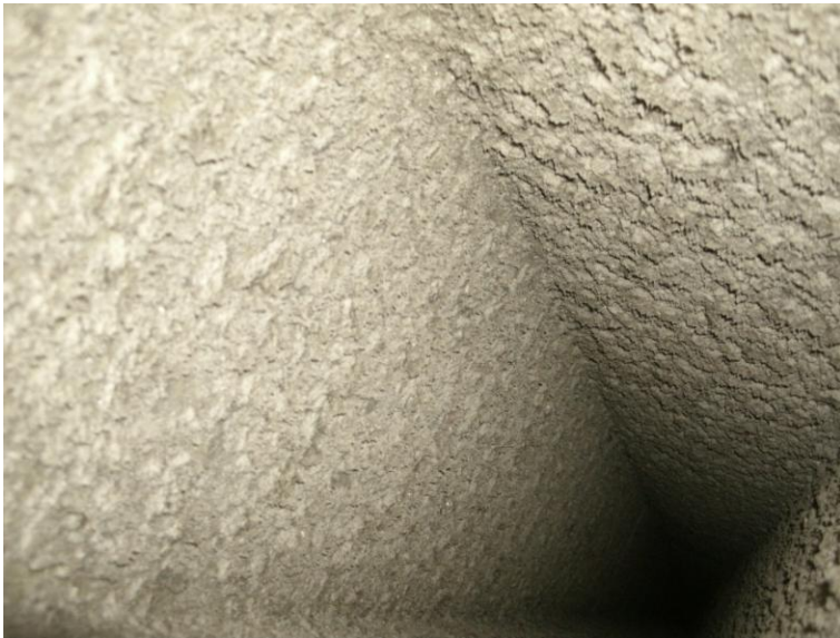
Very Dirty Shaft "Before" Cleaning
