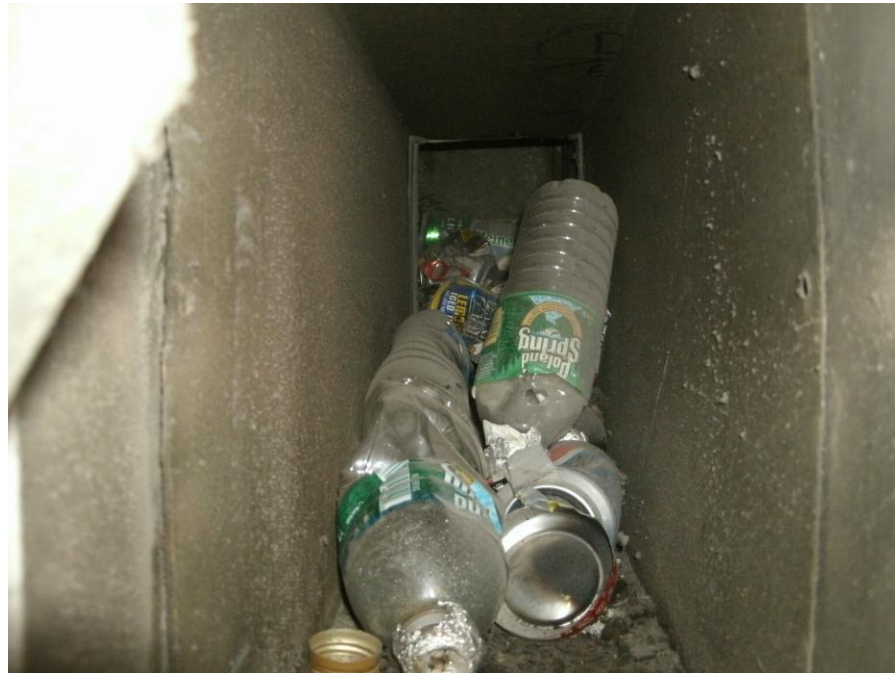
Exhaust Shafts are Often used as a Convenient way of Disposing of Debris During Construction
