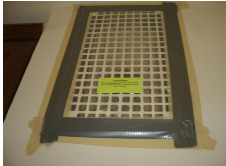
Vent Cover Replaced and Sealed Over w/ Plastic to Prevent Dust Intrusion During Shaft Cleaning
