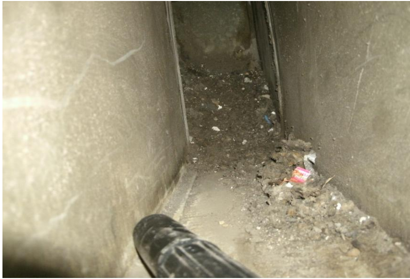
Dirty Vent Lateral at Bottom of Shaft "Before"
