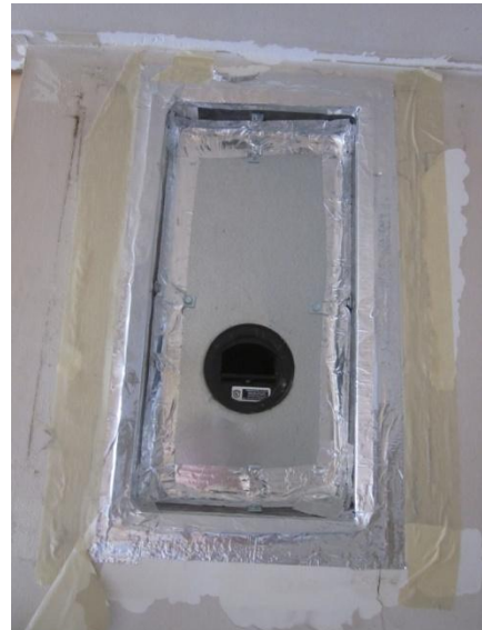
CAR Damper Assembly Installed and Sealed in Kitchen
