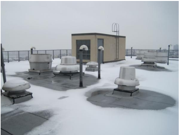
Roof exhaust fans. Note un-melted snow at non-working fans.
