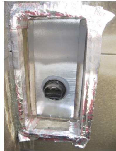
View from inside duct of sealed take off joint.
